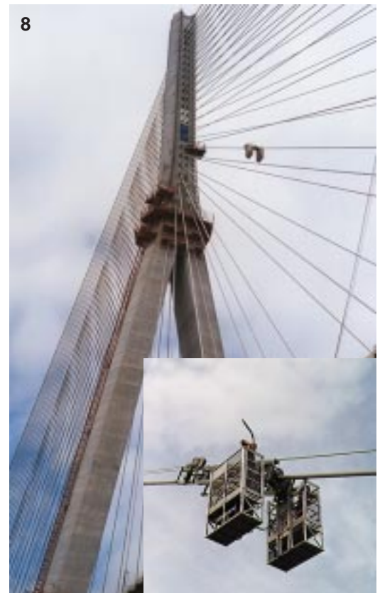
8 - Freely suspended cradle for inspection and maintenance of guy ropes on suspension bridge (Normandy Bridge). Powered TIRAK hoists and power pack mounted on the cradle.
