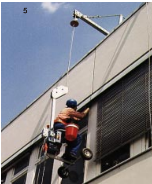
5 - The powered one-man lift SOLSIT is a particularly lightweight and economic solution for urgent repairs. Whether for ALTA platforms or for the SOLSIT, we recommend mobile roof rigs or parapet clamps. Sometimes an original solution is called for; we can do that.
